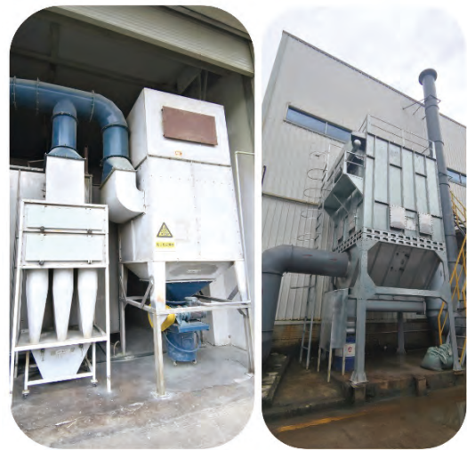
Exhaust air treatment facilities for painting and dust blasting process
