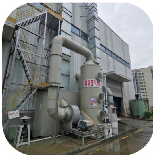
Alkaline liquid drip tower newly installed in Shenzhen plant
